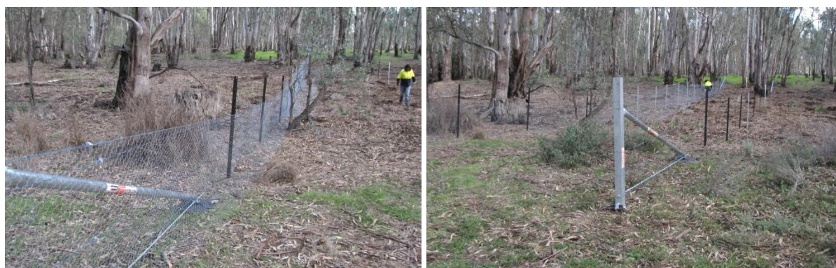
Figure 47 Exclusion fence (left) and accompanying debris fence (right) constructed on a major flood runner leading into Reedy Lagoon, May 2014.
