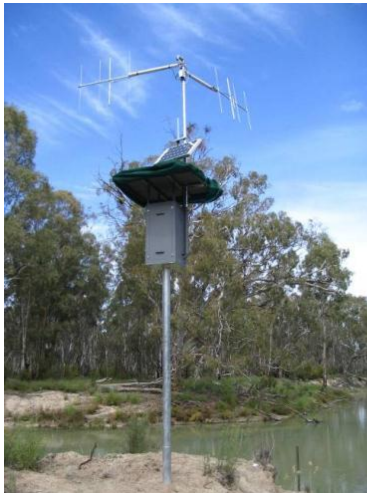
Figure 5. Upper Mullaroo data logger, showing logger box, solar panel and antennae.
