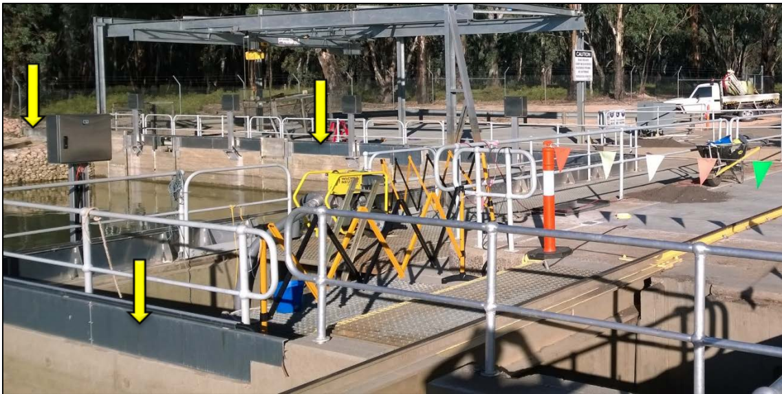
Figure 6. Fishway 'barrier' (indicated by yellow arrows) at Lock 8, which runs the perimeter of the fishway structure and extends into the rock levee bank at the far left (photo: Karl Pomorin).
